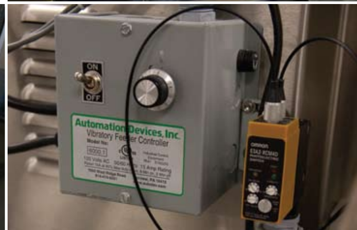
The vibratory feedins system working with the JDA Pro-Cap 5000 capper incorporates several Omron photoelectric switches.
